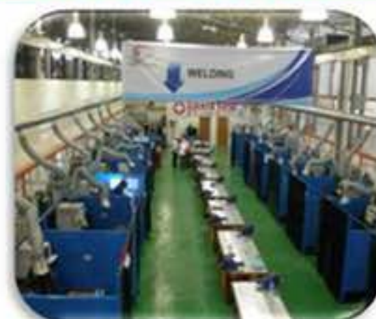
Classroom Fume Extraction System
